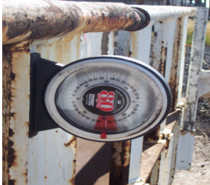
Fig 17 – Magnetic Inclinometer attached to Bretby. Panline LW103
